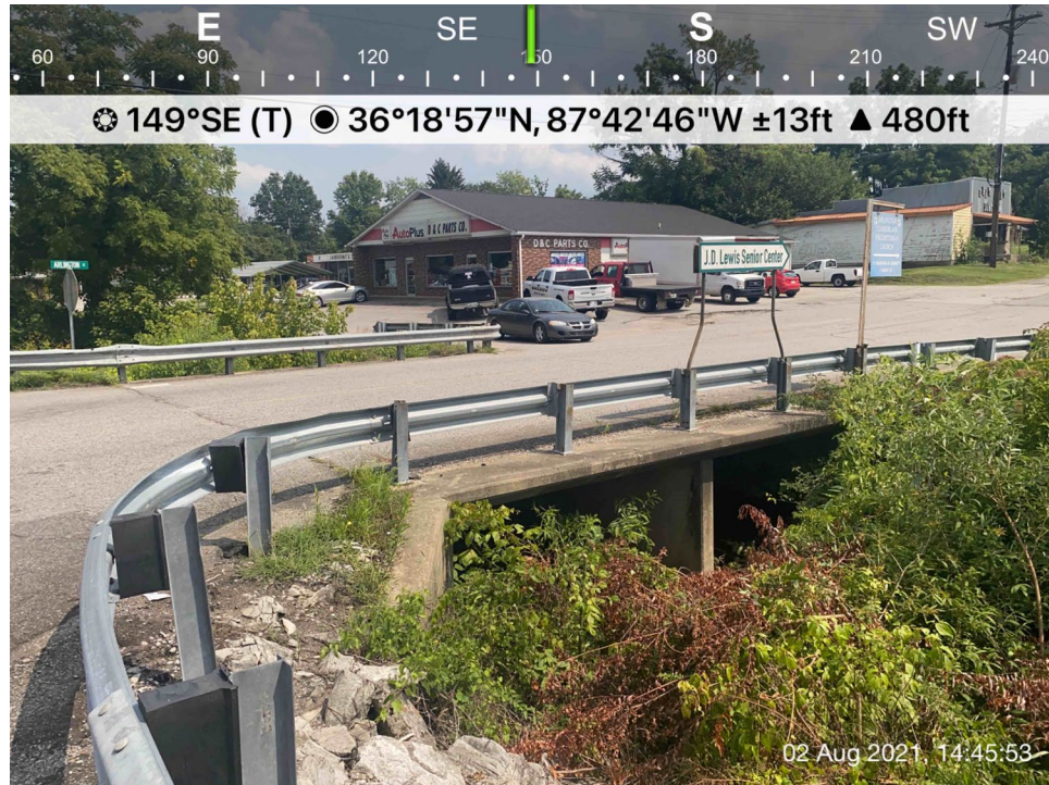
Figure: View of bridge from southern ROW of SR-49, west side of T-intersection
